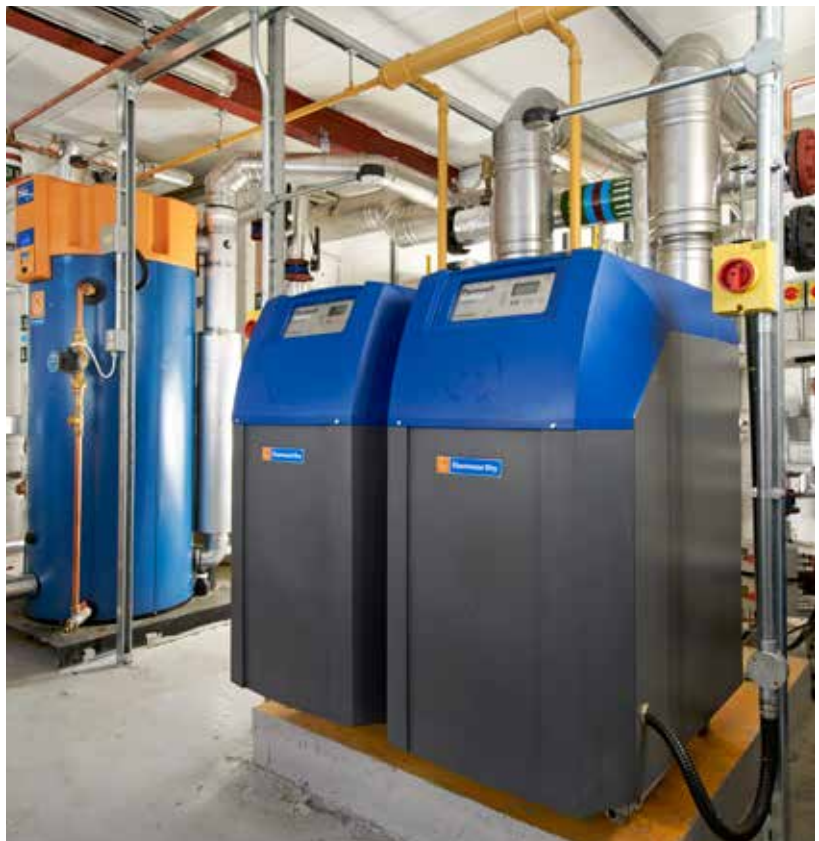
Typical plant room with Purewell VariHeat high efficiency condensing boilers and a Dorchester DR-FC Evo condensing water heater.
